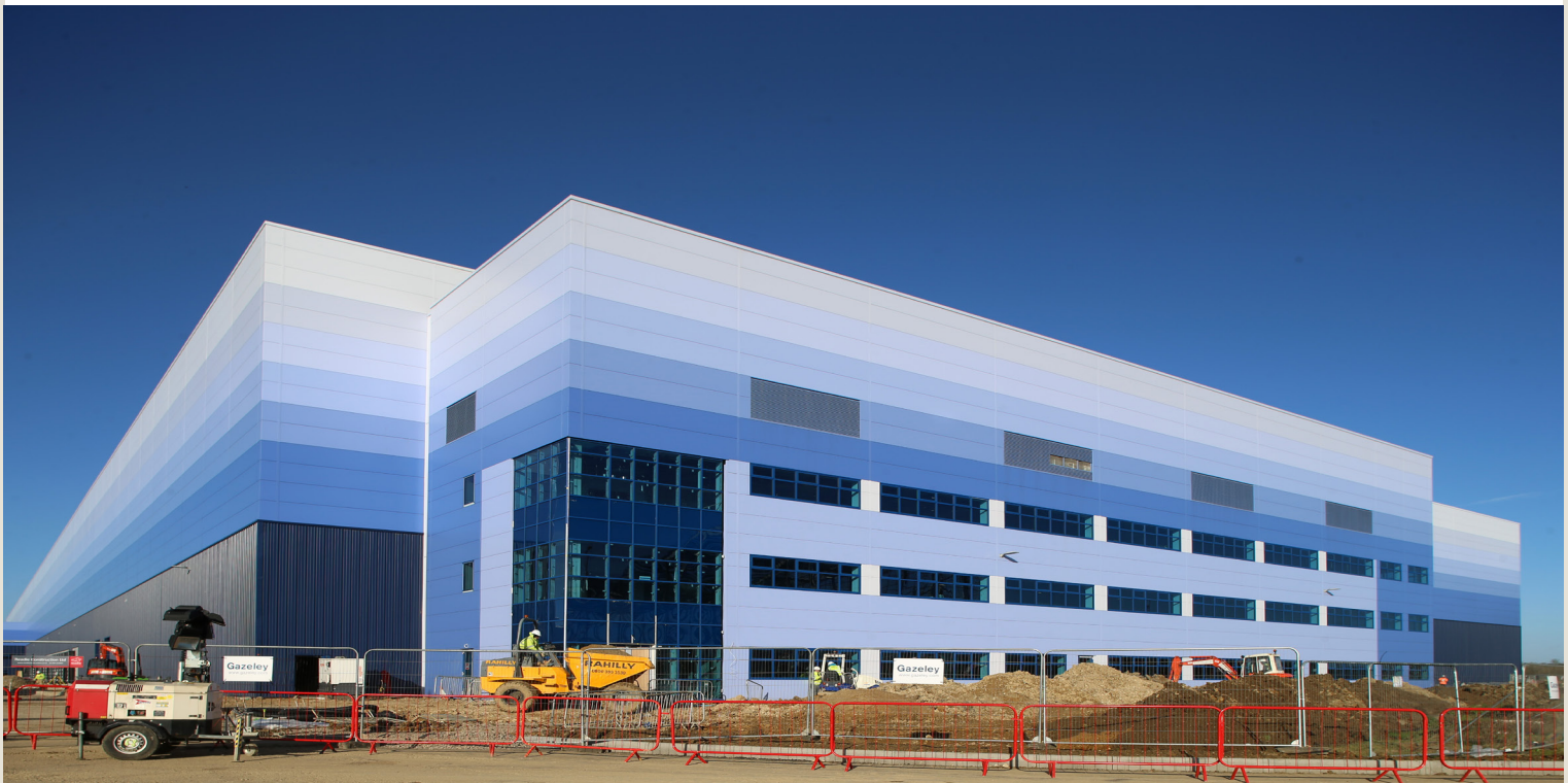
Altitude Milton Keynes where a unit of 574,000 sq ft is being developed by Gazeley and due to complete in the first quarter of 2018
